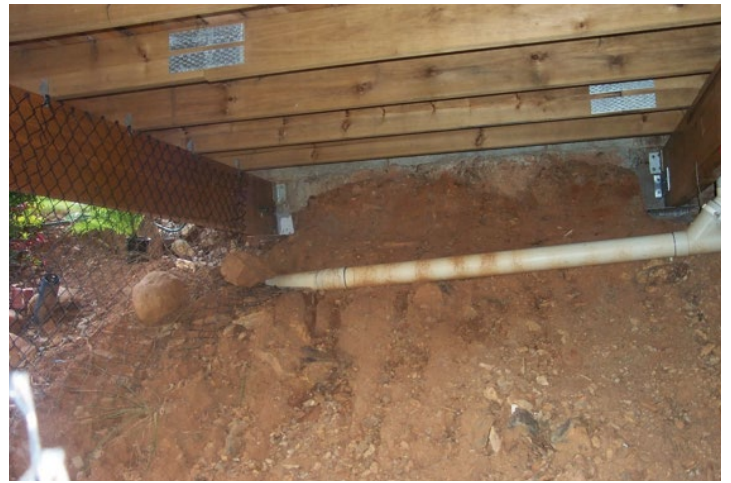
Photograph 4 - NOT ACCEPTABLE – Uncoated Z275 nail plates and framing anchors in Low Hazard Zone but Exposed Condition under a deck.
