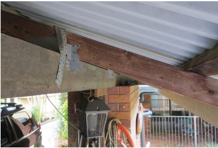
Photograph 1 - ACCEPTABLE – Z275 bracing, multigrips and truss plates in a Low Hazard (>10km from surf) Sheltered Condition. Note: Connectors have been installed for 35 years.
