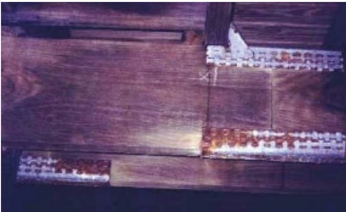
Photograph 3 - NOT ACCEPTABLE – Z275 connectors in deck joists 1 km from surf. 6 years old, Sunshine Coast.
