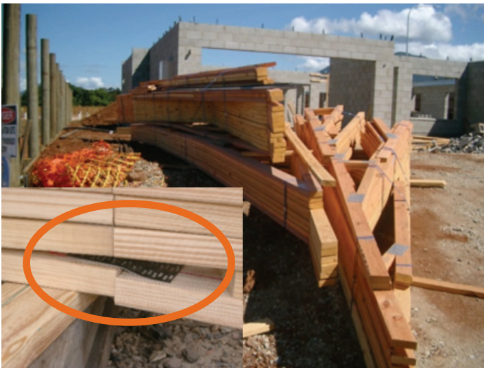
Photograph 1 – Don't install site damaged trusses or those with manufacturing faults. Replace or repair before erecting
