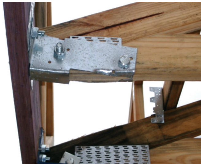
Photograph 7 – Girder brackets not installed correctly
