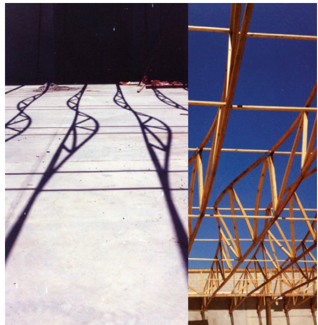
Photograph 10 – A pronounced example of incorrect installation leading to trusses being twisted and out of plumb
