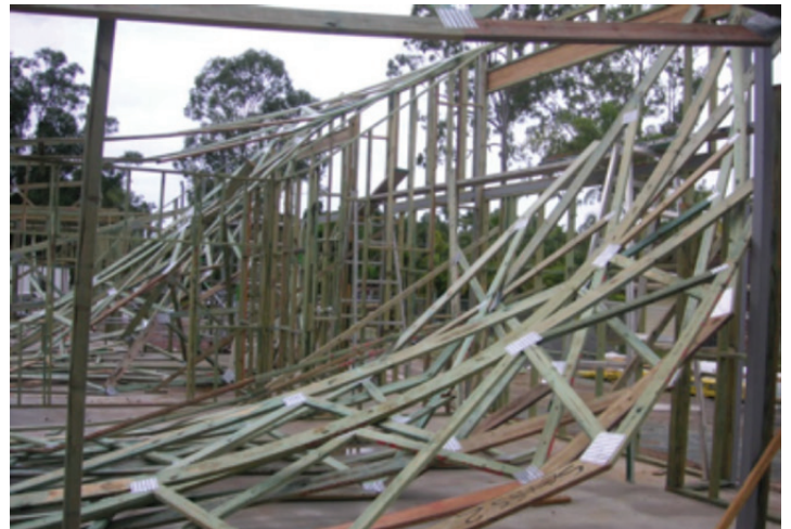
Photograph 4 – Dangers of not providing temporary bracing
