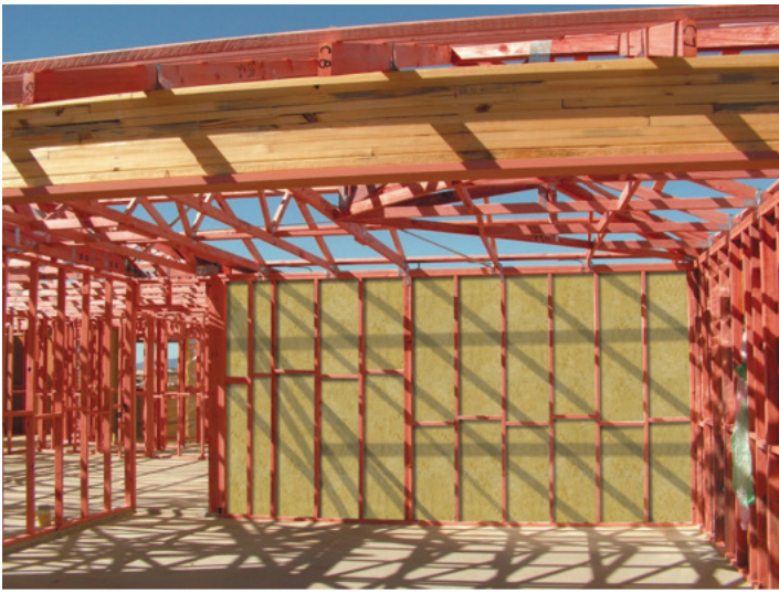
H2 termite treated structural softwood framing.
